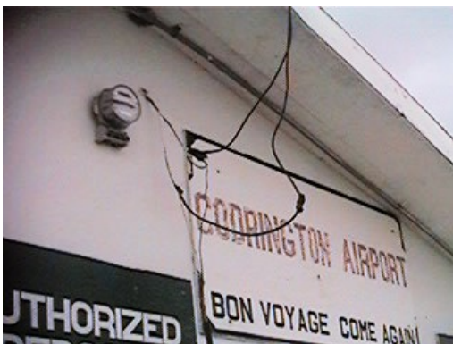
Figure 7 typical electricity meter
