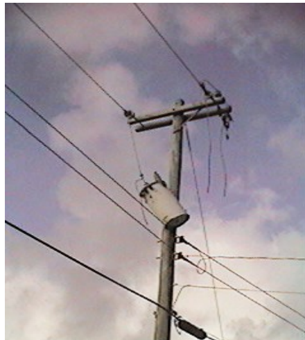
Figure 8 local transformer 4,000v-220v
